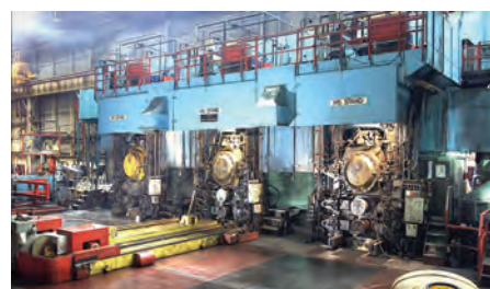
Parkegate are dismantling the 3-stand, hot finishing mill at Rogerstone to substantially upgrade to as new condition
